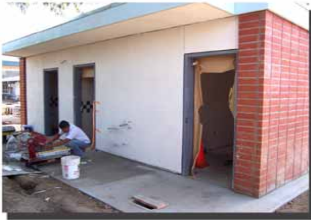
WORK IN PROGRESS FOR NEW STAFF RESTROOMS, ELECTRICAL, & JANITORIAL ROOMS IN BUILDING "R"
